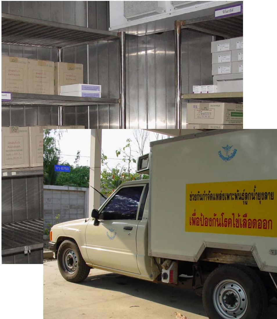
EPI Cold room in Chon Buri
